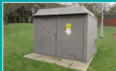
Example of a typical substation that serves residential/commercial properties with electricity
