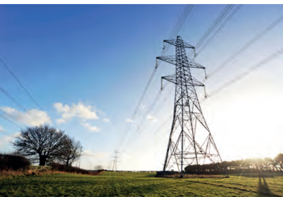
Example of an electricity pylon
