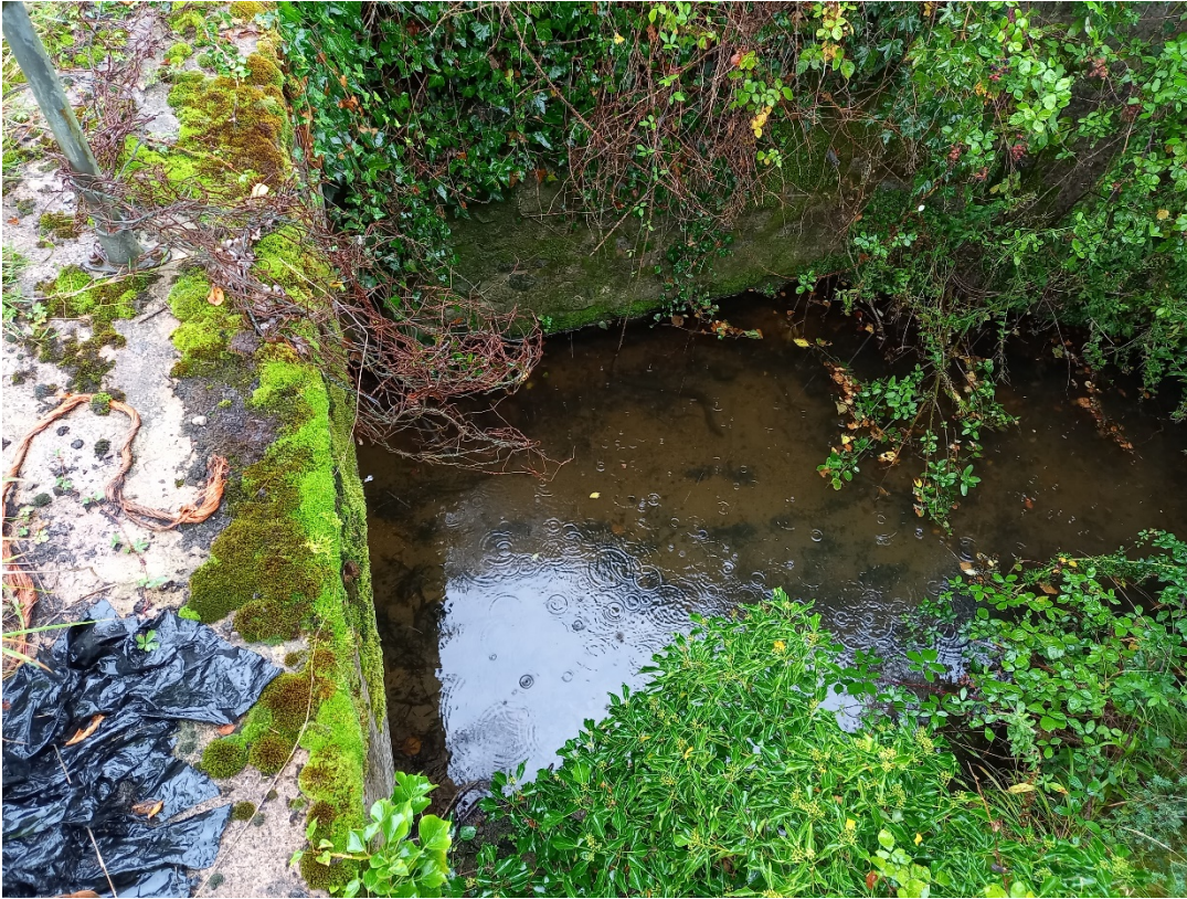
Figure C-13 Site 30 DS Impacted
